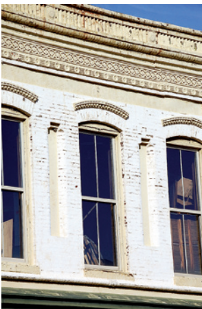
Brick is the dominant exterior material in the commercial section of the Franklin Historic District. As with residential buildings, the exterior material both protects the structure and expresses architectural style.
