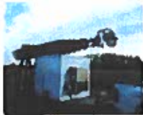
106' TowerWorx with Shelter & Generator
